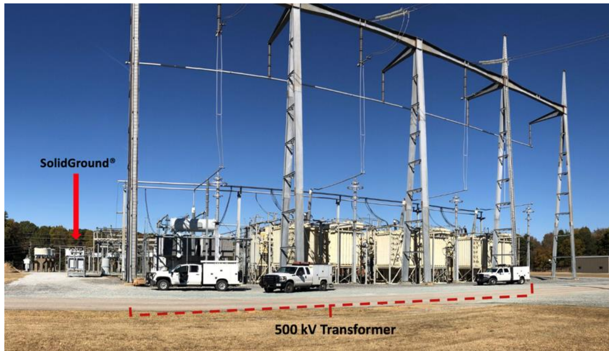
“SolidGround” protecting a 500KV transformer in the TVA grid.
