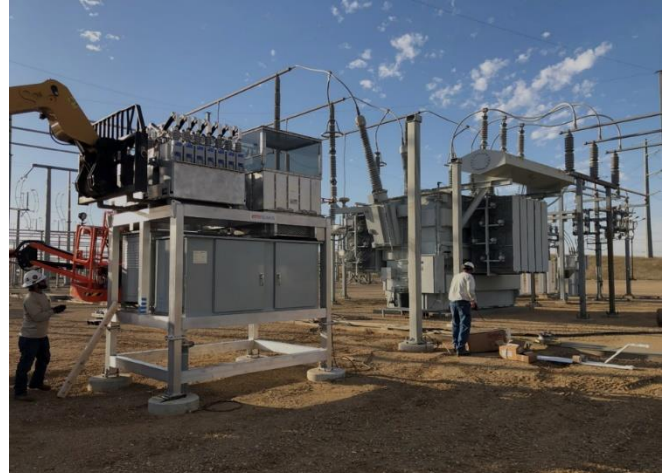
“SolidGround” being installed on DOE’s 345KV transformer in the WAPA grid in South Dakota.
