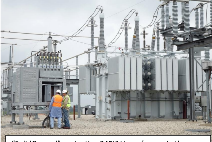
“SolidGround” protecting 345KV transformer in the ATC grid in Wisconsin (9+ years of testing)
